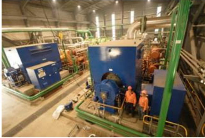
This is the turbine hall of CSR's $150 million Pioneer Sugar Mill cogeneration facility commissioned in 2006. The opportunity for more such facilities across the sugar industry could be lost if taxation-favoured forestry continues to intrude on commercial sugarcane farming operations.
