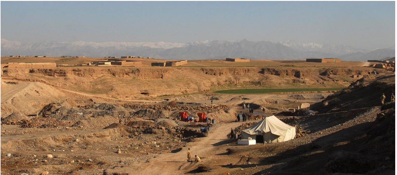
The construction site of the eastern causeway bridge in Tarin Kowt, one of many projects designed and project managed by the Australian 1 st Reconstruction Task Force. (image courtesy of the Department of Defence)
