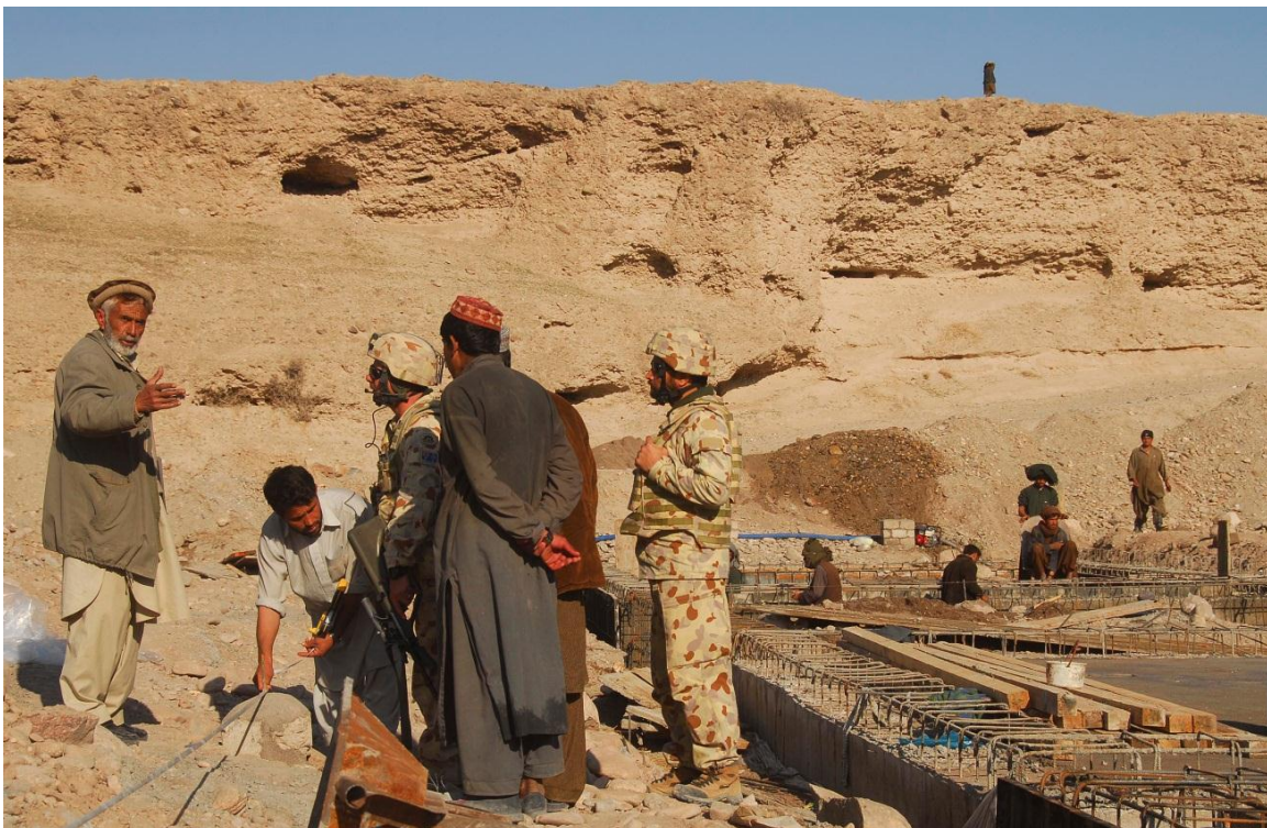
Australian 1st Reconstruction Task Force soldiers consult with local Afghan contractors about the progress of the eastern causeway bridge. (image courtesy of the Department of Defence)
