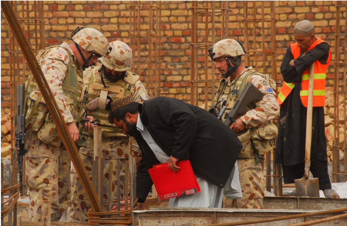
Australian 1st Reconstruction Task Force soldiers receive an update from the local contractor on the progress of a new government building during a site inspection. (image courtesy of the Department of Defence)
