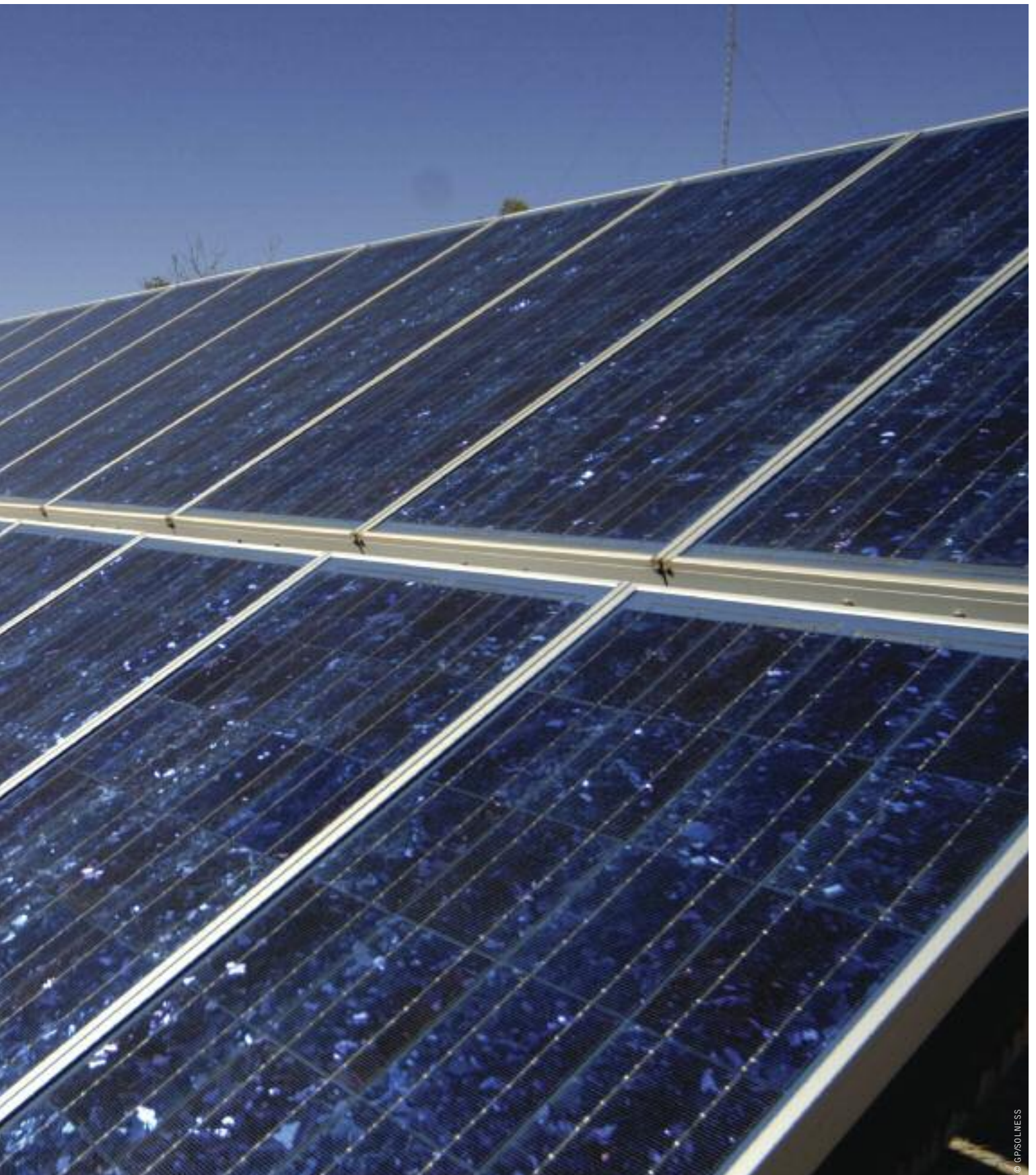
image SOLAR PANELS ON CONISTON STATION, NORTH WEST OF ALICE SPRINGS, NORTHERN TERRITORY.
