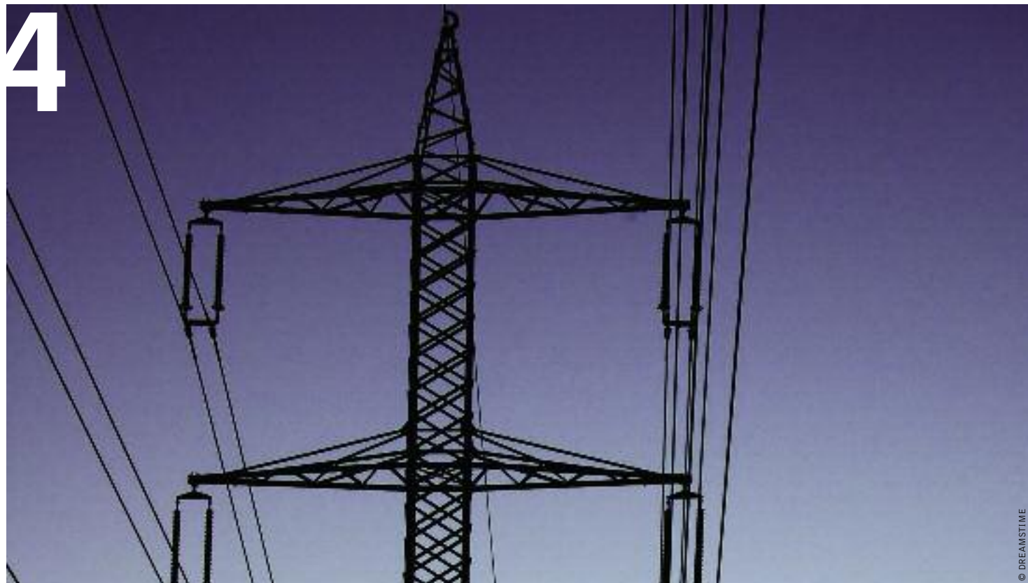
image ELECTRICITY LINES.
