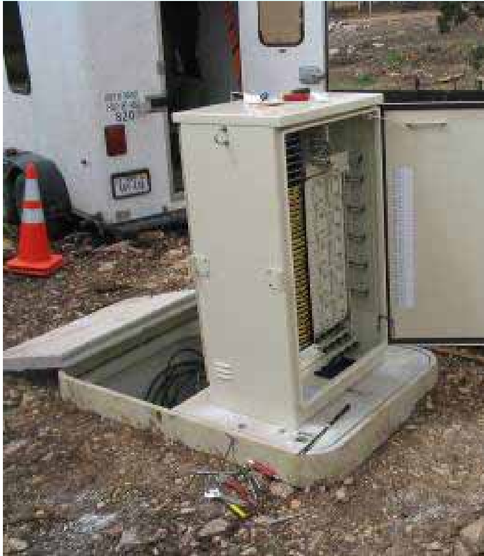
Underground optical termination enclosure
