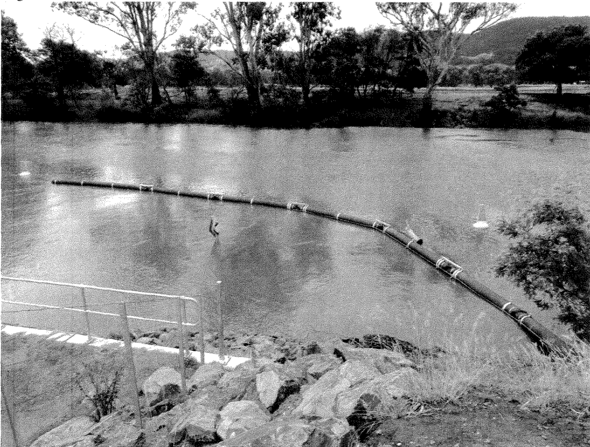
The intake on the Goulburn River for Melbourne and its North South pipeline-just in front of the house that is the pump shed! Photos by Maria Riedl November 2010.
