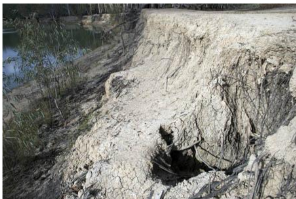
Erosion on river banks;
