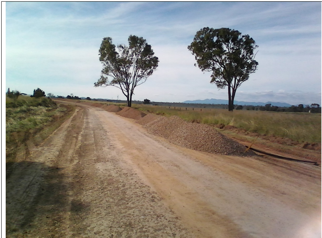
Figure 1. Gravel top dressing on road in the Fitzroy catchment of central Queensland. This was a continuous line of dumped material for 2km of a 4km stretch of road.
