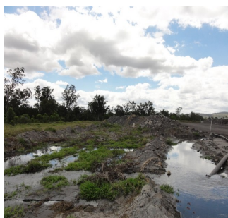
At 10.30am 13.9.10 the site was inspected by SMM superintendent, and there was evidence that water had spilled from the drainage channel, and had made it's way under a drainage bund between the channel and the levee (piped through a crack in the bund), and drained over the levee towards the creek.
