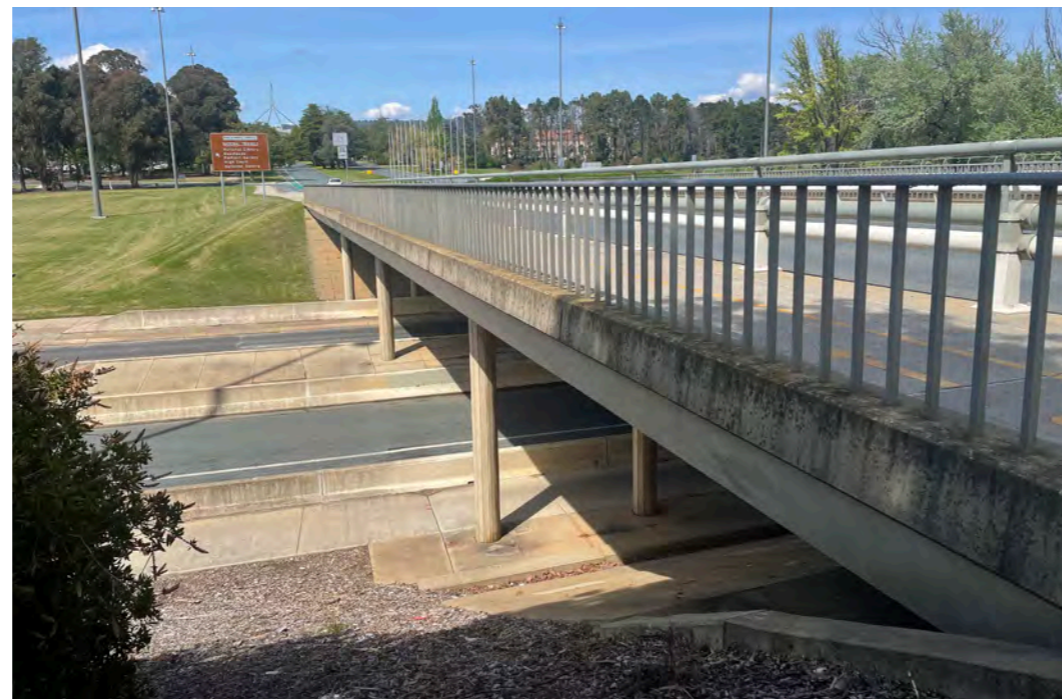
Figure 162: Flynn Drive Bridge detail.
