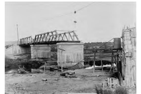
Figure 29: 1928. The original Commonwealth Avenue Bridge under construction. Source: National Archives of Australia, A1200, L83799, Item ID 11777528.
