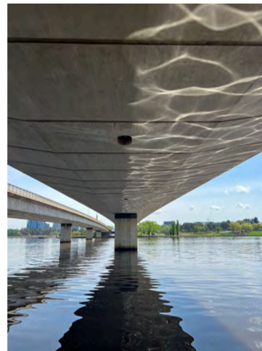
Figure 172: Soffit of southbound bridge showing hole with lighting.
