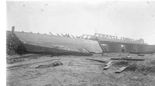
Figure 16: 1925. Second Commonwealth Avenue Bridge showing embankment form work. Source: National Archives of Australia, A3560, 1224, Item ID 3118731.
