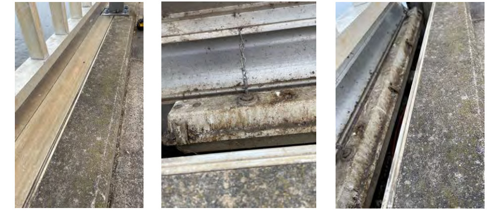
Existing CAB access to parapet panel lighting
