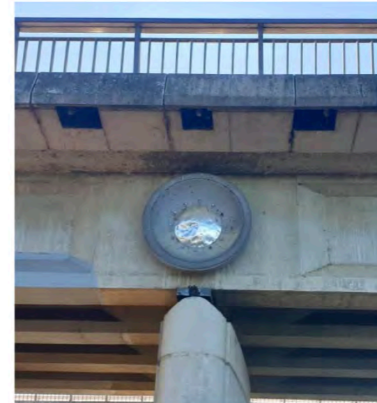
Figure 3.4 Kings Avenue Bridge lighting in handrail and below to light roundel. (Source: K Baker, 2020)
