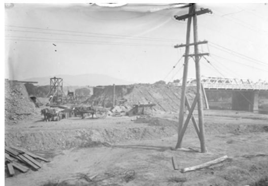
Figure 21: 1926. Commonwealth Avenue Bridge embankment under repair following 1925 floods. Source: National Archives of Australia, A3560, 1422, Item ID 3120825.
