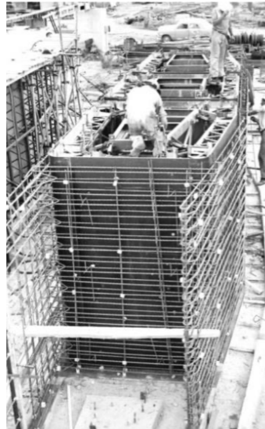
Figure 59: Reinforcement placed around inner form of box segment. Source: National Library of Australia, nla.obj 24577602
