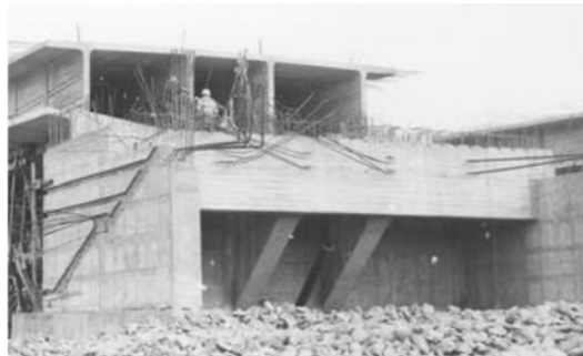
Figure 53: 1962-63. Bridge abutment, supporting an end span of the superstructure. Source: National Library of Australia, nla.pic-an24577607-v
