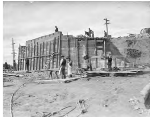
Figure 22: 1926. Commonwealth Avenue Bridge embankment. Source: National Archives of Australia, A3500, 1715, Item ID 3130215.
