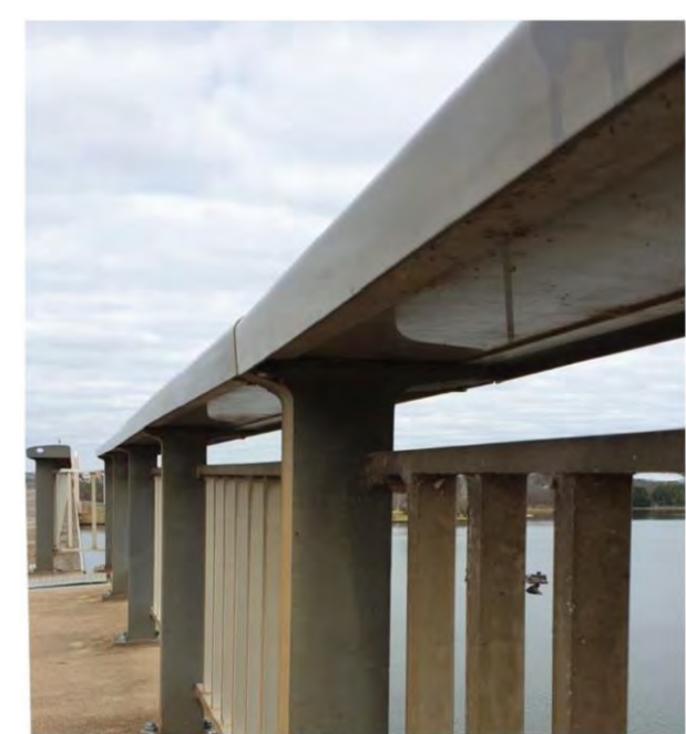
Figure 3.7 Detail of integral handrail lighting of the Commonwealth Avenue Bridge. (Source: K Baker, 2020)
