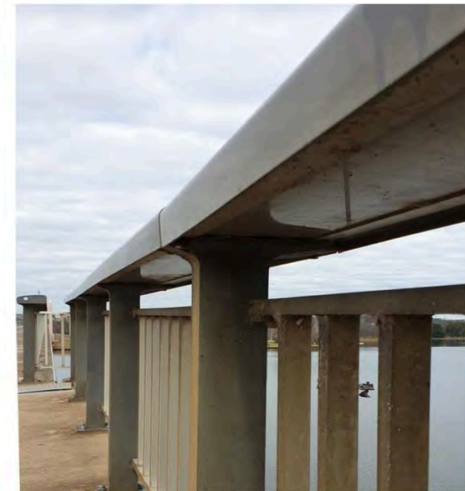
Figure 3.7 Detail of integral handrail lighting of the Commonwealth Avenue Bridge. (Source: K Baker, 2020)
