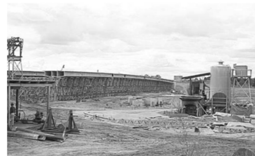
Figure 61: Multi-webbed box segments in place on top of the timber falsework. The concrete batching plant and casting yard are in the foreground. Source: National Library of Australia, nla.obj-143758146-1
