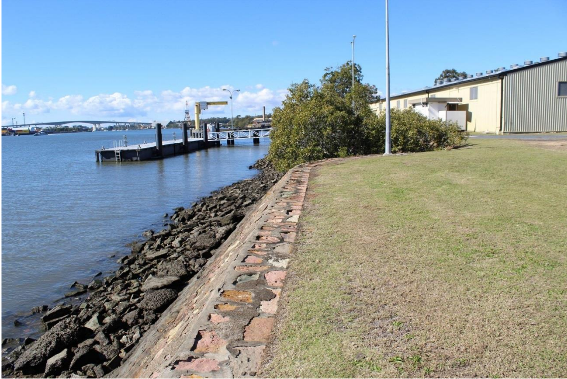
Figure 35: Section of sea wall that will have 2 water pipes inserted to assist storm water drainage from the site. (GML 2017)
