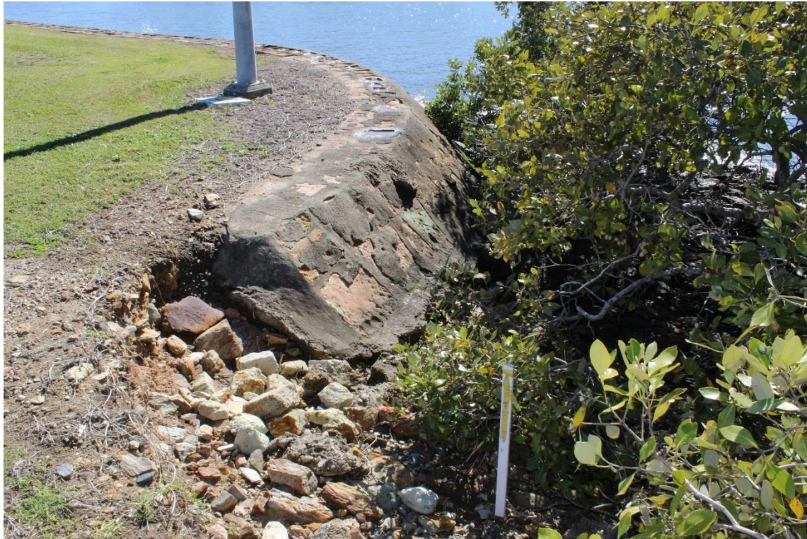
Figure 37: Detail of sea wall and gravelled break in the sea wall interface on the western side of the break. Minor works will be required to the sea wall to integrate the proposed boat ramp. (GML 2017)
