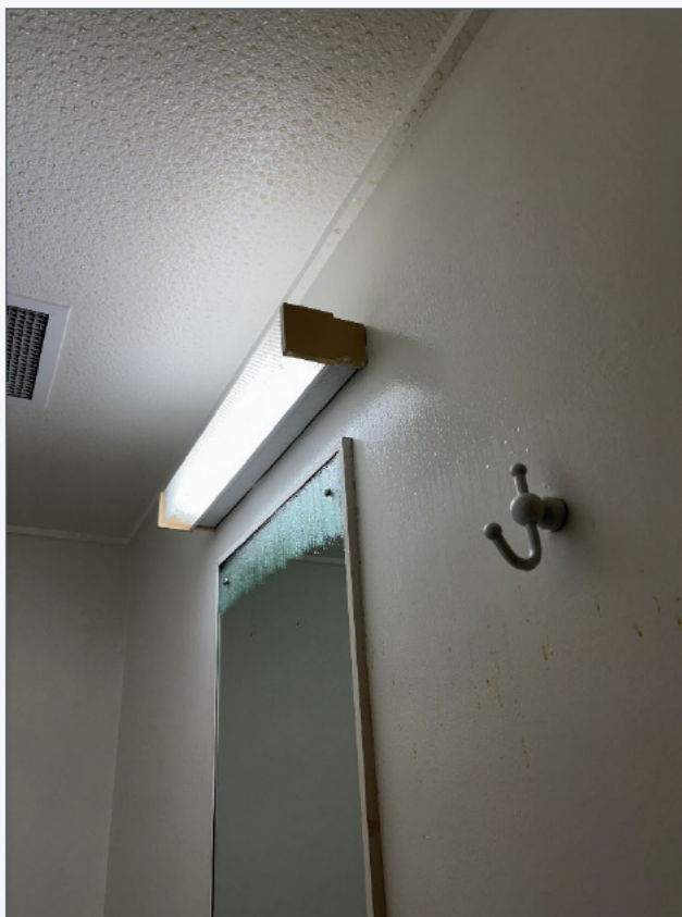
The causes of condensation are multifaceted and require remediation.
