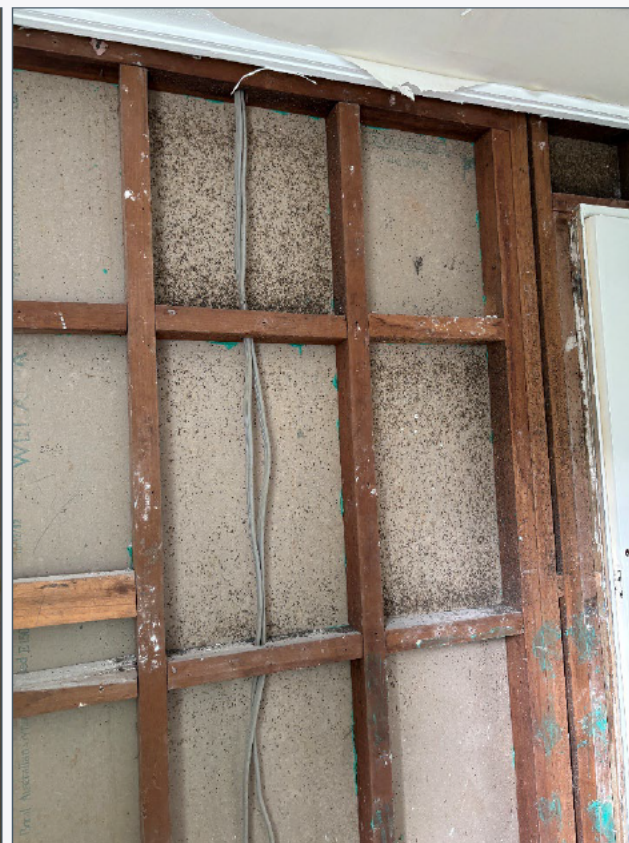
Undisturbed mould within concealed spaces behind fixed linings.
