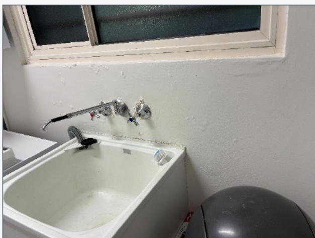
Aging finishes and typical water damage around sills.
