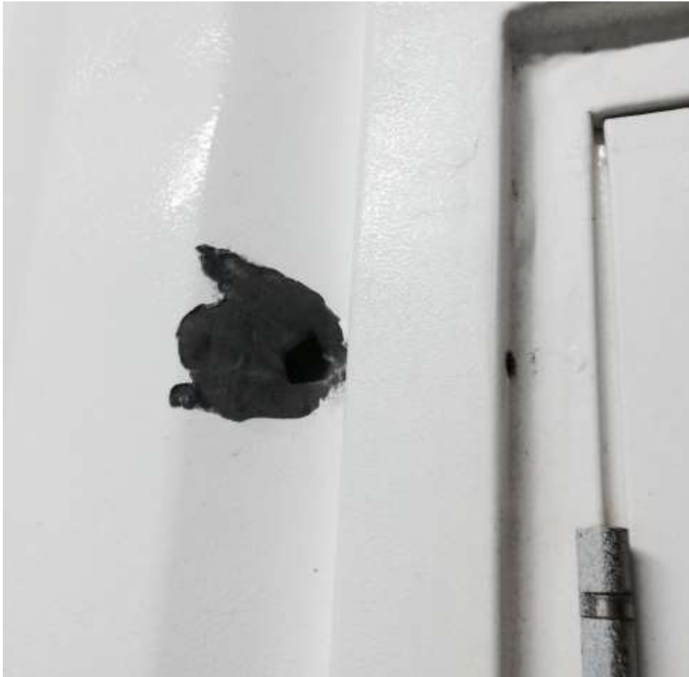
A bullet hole in a wall at Manus Island Immigration Detention Central following an incident between February 16 and 18, 2014. Image supplied 1 May 2014. © AAP Image/Supplied
