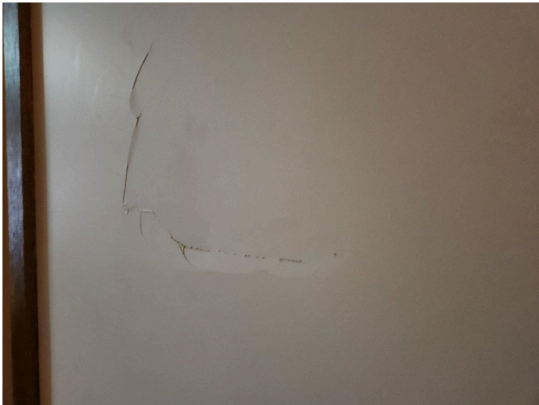
One of many wall impact sites throughout the home. This damage remains unrepaired. August 2025.
