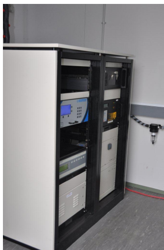
Ammonia, NOx and NO2 Monitor
