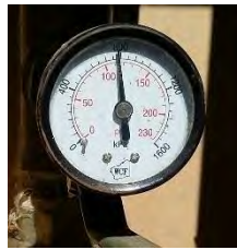
Photo taken at 4 th monthly inspection 5.5.17 – 800kpa pressure in fire system on arrival
