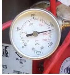
Photo taken at 5 th monthly inspection 1.6.17 – 1300kpa pressure in fire system on arrival
