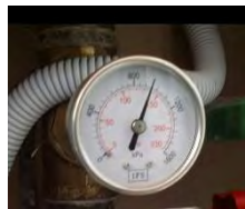
Photo taken at 3 rd monthly inspection 5.4.17 – 950kpa pressure in fire system on arrival
