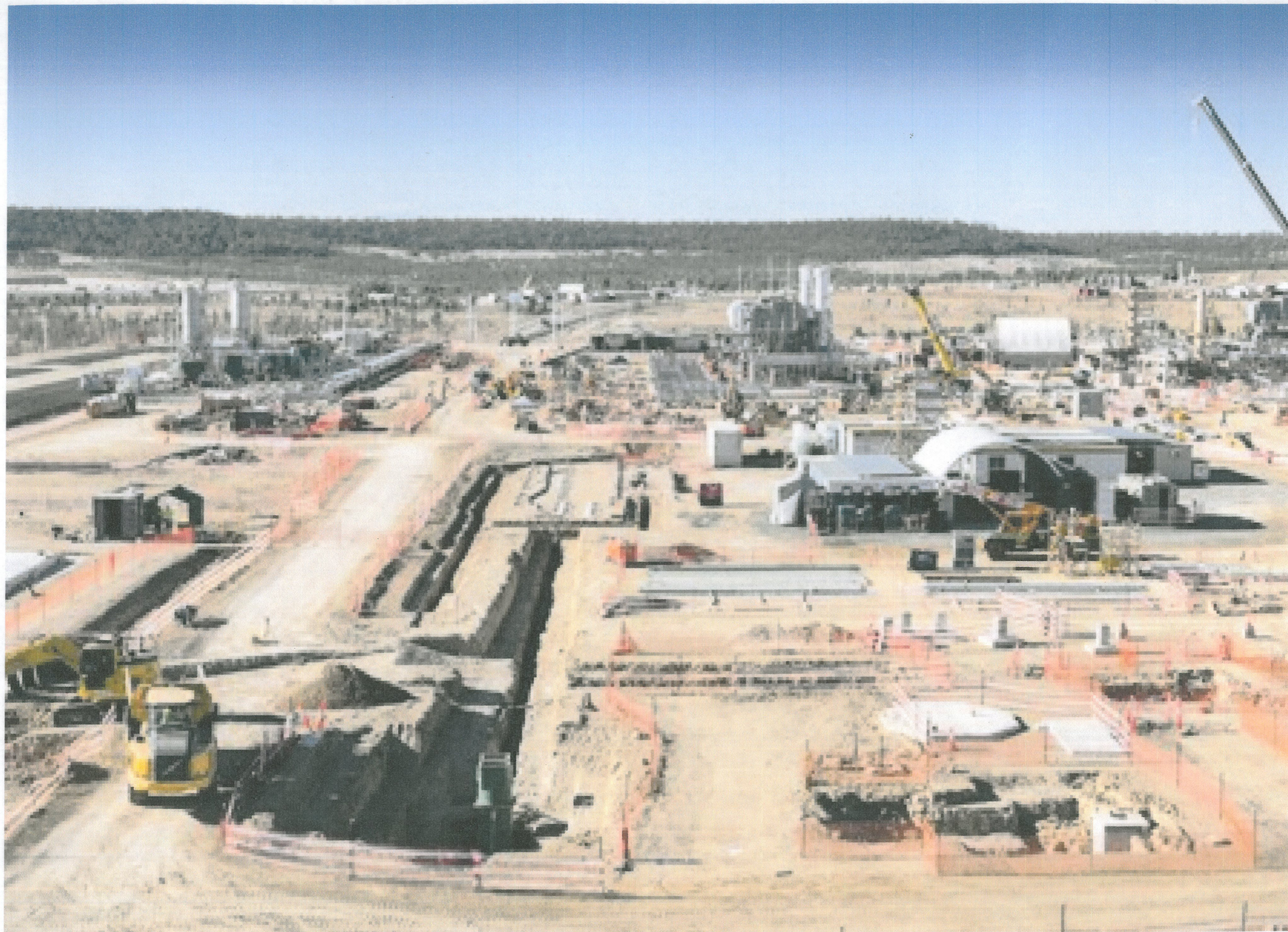
Underground services are installed in trenches in the utilities area at the smaller of two gas hubs in Fairview field. Concrete foundations will soon be poured for other facilities set to be built in this area.
