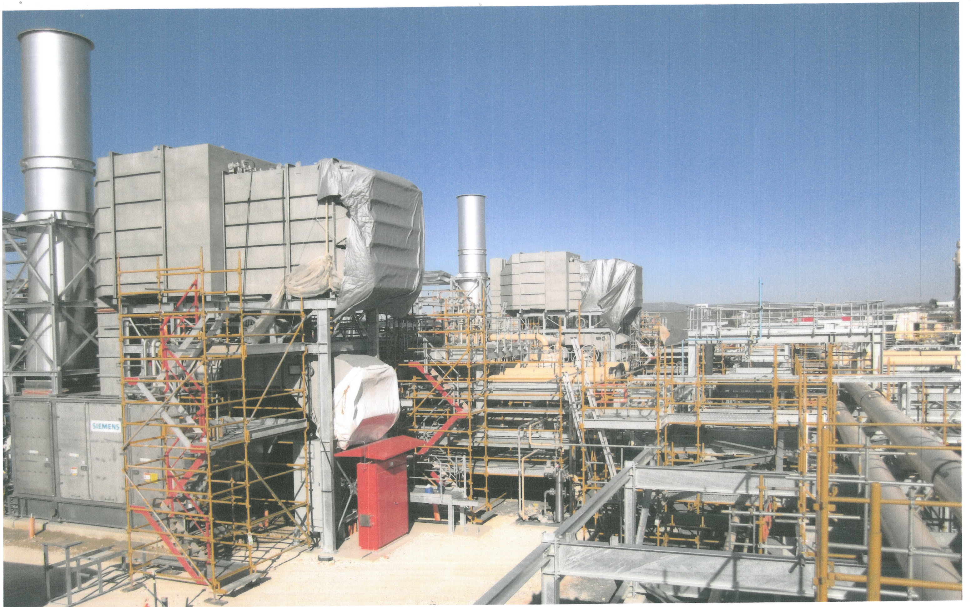
Gas turbine compressor piperack in the hub compressor station area at Santos GLNG's Roma hub, one of three gas hubs under construction.
