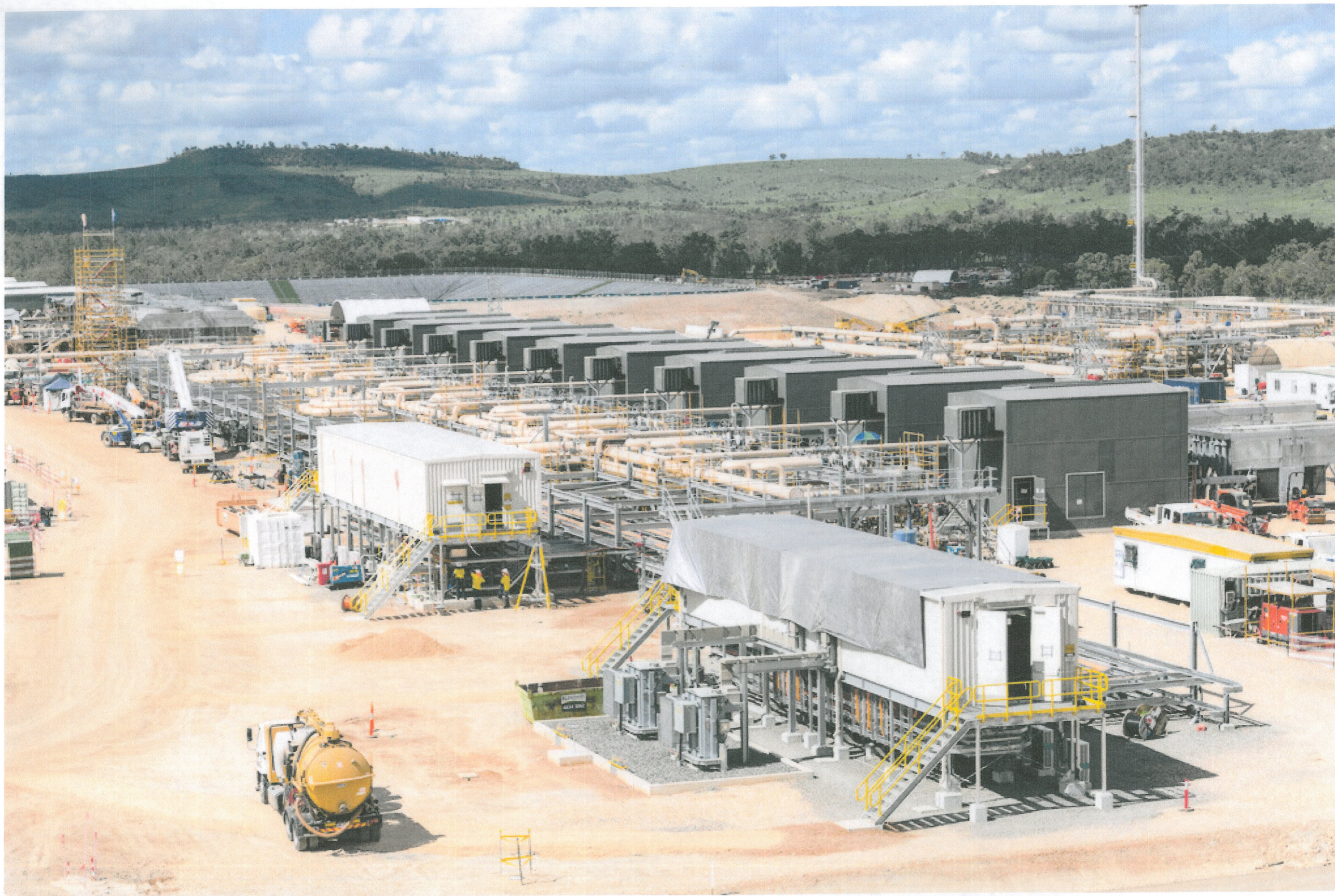
Electrical connections are underway for the nodal compressors at Fairview Hub 04 in Fairview field
