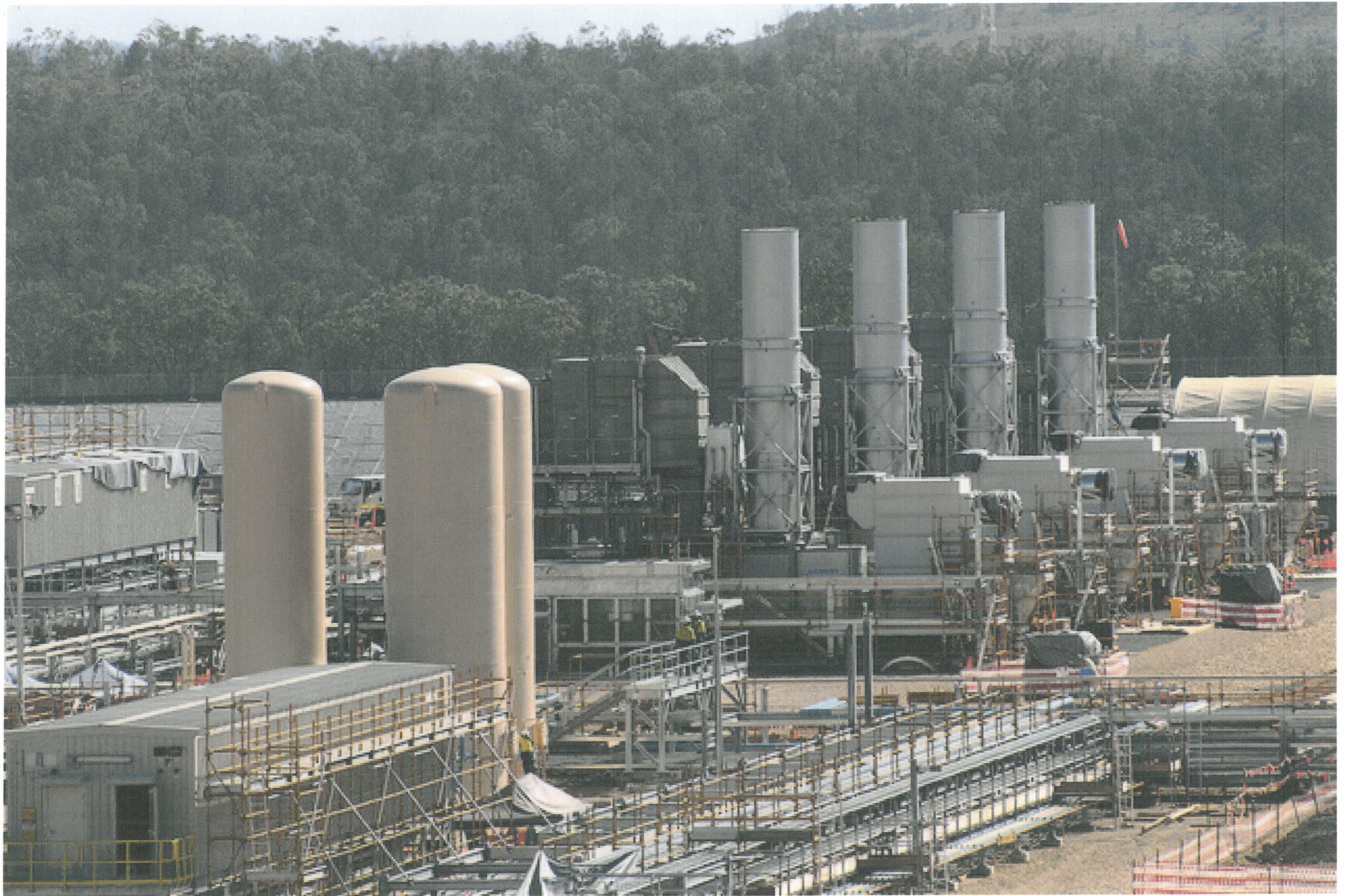
Gas turbine compressor piperack in the hub compressor station area at Santos GLNG's Roma hub, one of three gas hubs under construction.
