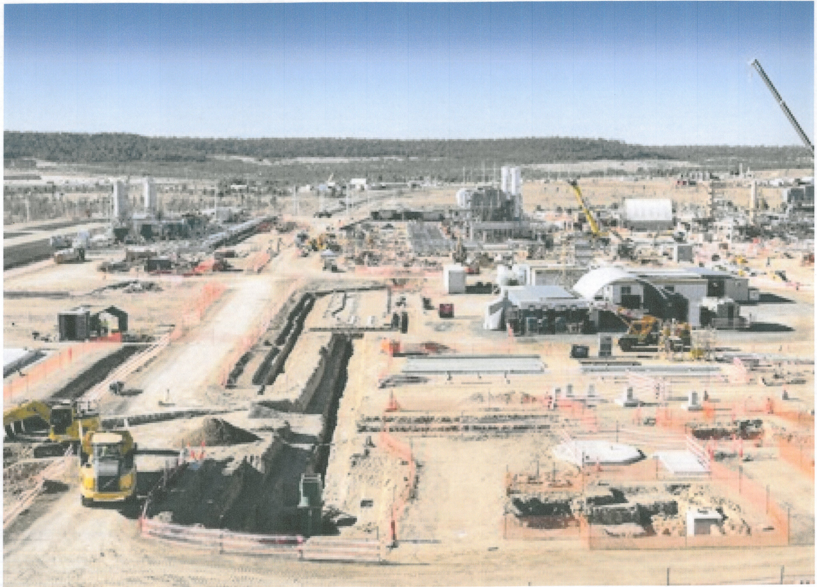
Underground services are installed in trenches in the utilities area at the smaller of two gas hubs in Fairview field. Concrete foundations will soon be poured for other facilities set to be built in this area.
