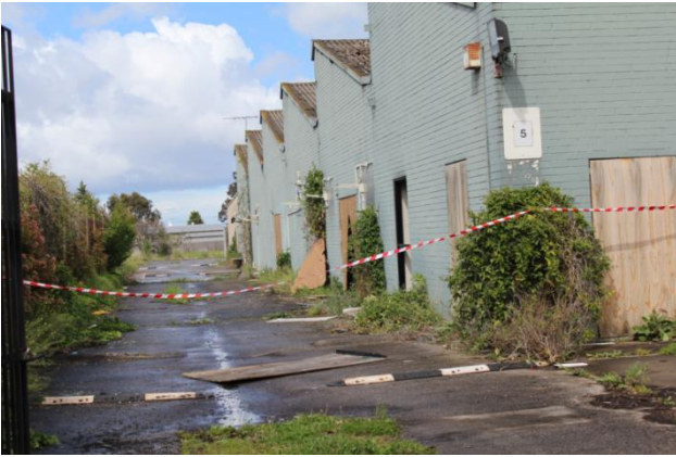
Abandoned Yakka site recently set alight.
