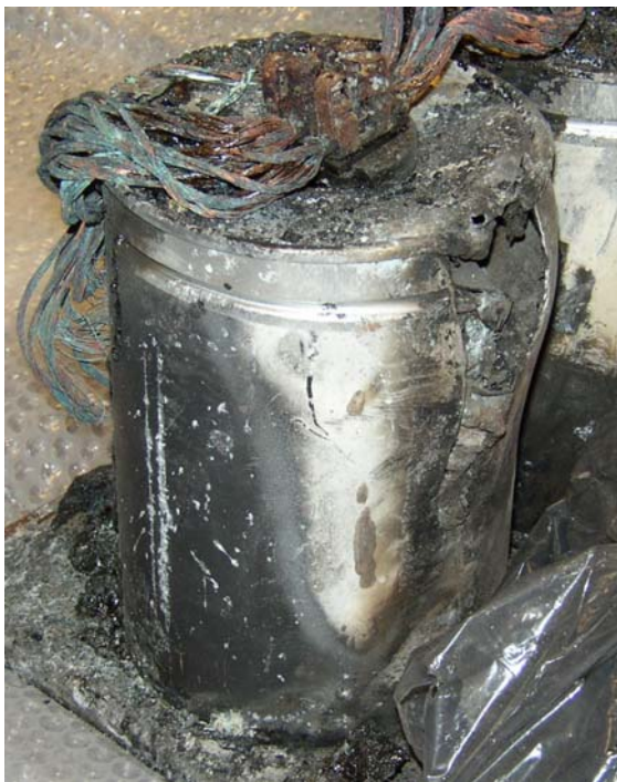
Fig. 4: Burst pressure vessel of a line filter capacitor (Image source: Allianz)
