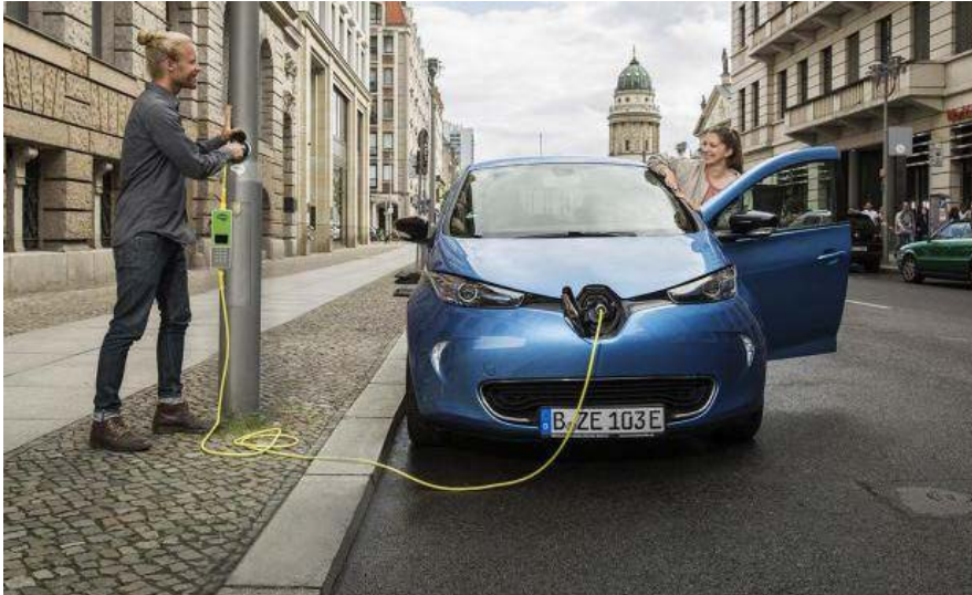
Figure 48: Street Light Charging Socket (Source: Ubitricity)
