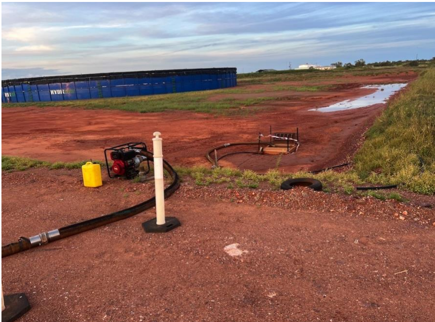
6 Hydrera Water treatment plant pumping contaminated sump water over bund wall, site entirely accessible.
