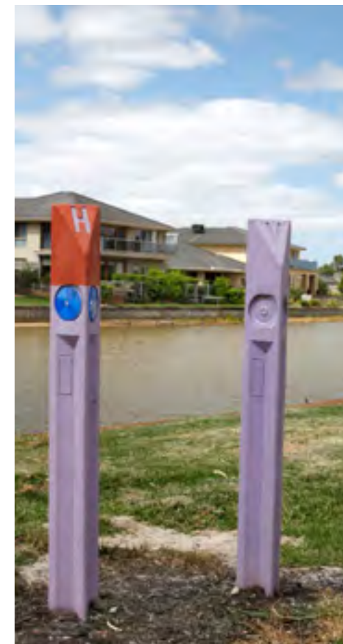
Above The Sandhurst Club, located just outside of Frankston in Melbourne's south east, uses purple pipes and recycled water to reduce its dependence on mains water supply
