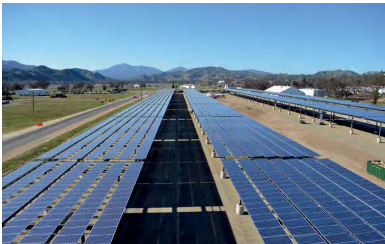
Figure 46: Solar panel arrays at Fort Hunter Liggett, in California. Fort Hunter Liggett was selected by the US Army to be converted to a net zero energy base.
