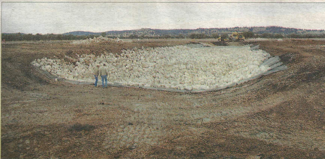
Mullaley Gas Pipeline Accord (MGPA) members, David Quince and Wal Warden, inspecting the massive pipeline reconstruction works at Peter and Charmaine Cook's property.
