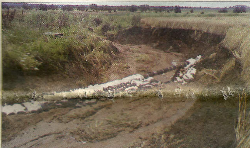
The Central Ranges gas pipeline exposure on Peter and Charmaine Cook's farm, north of Coolah.
