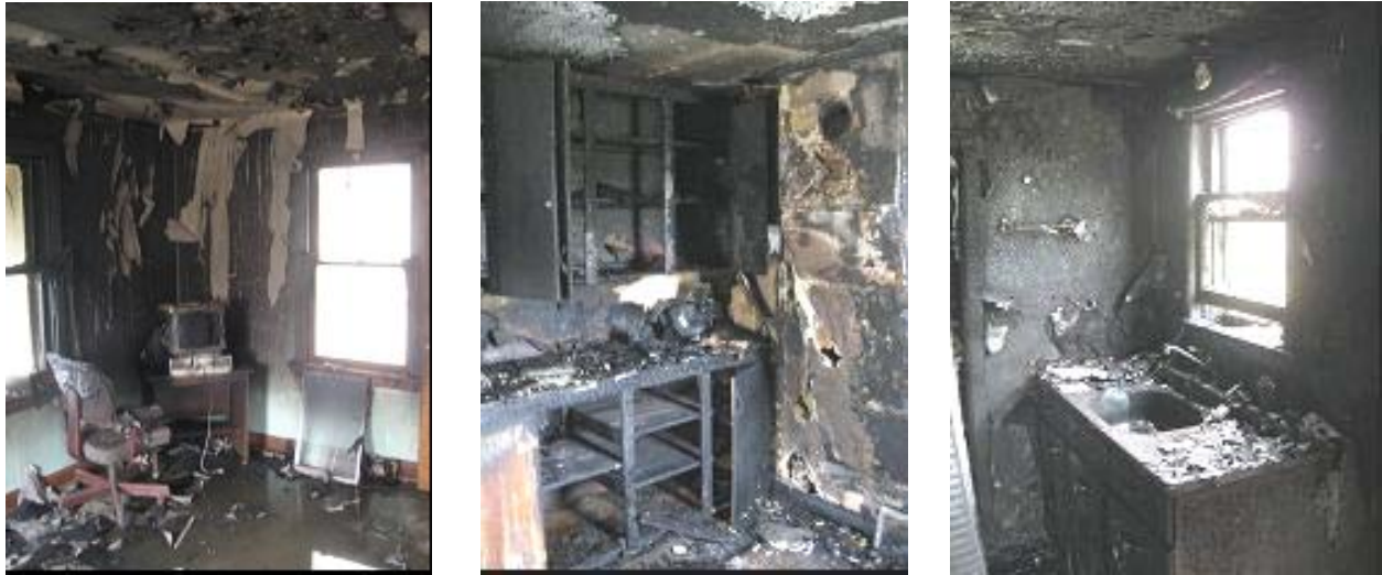
Figure 5-10: Kitchen after the controlled field fire event.
