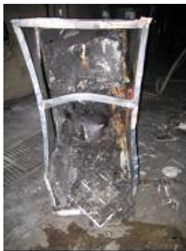
Refrigerator (post fire)
