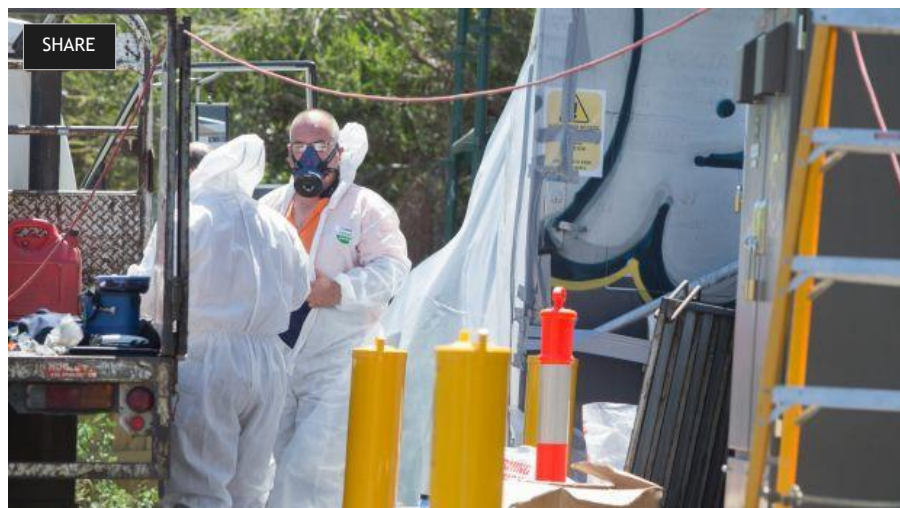
Workers prepare to remove asbestos from the substation in Thornbury. Photo: Simon Schluter
