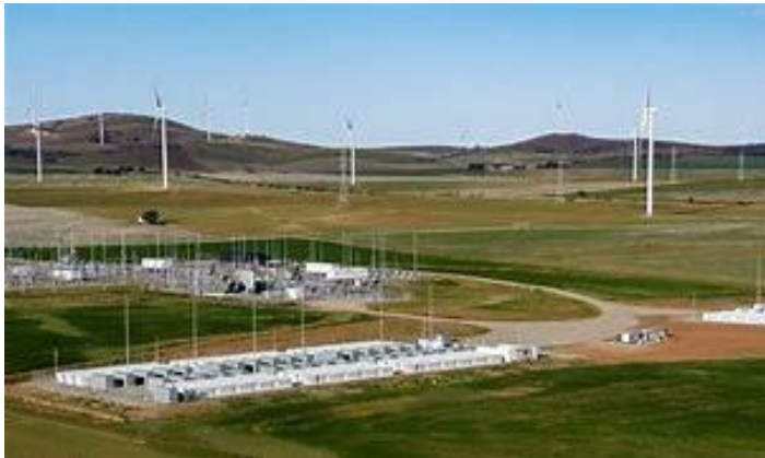
Hornsdaile Power Reserve (batteries) and Wind IEGW, South Australia
