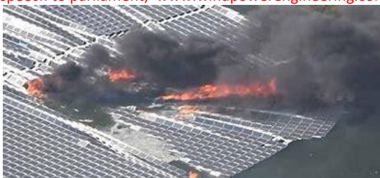
PV solar IEGW left to burn out
