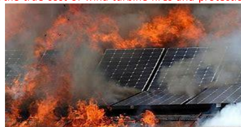
PV solar panel fire
