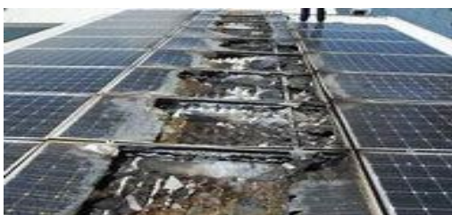
Fire shuts down whole solar array
