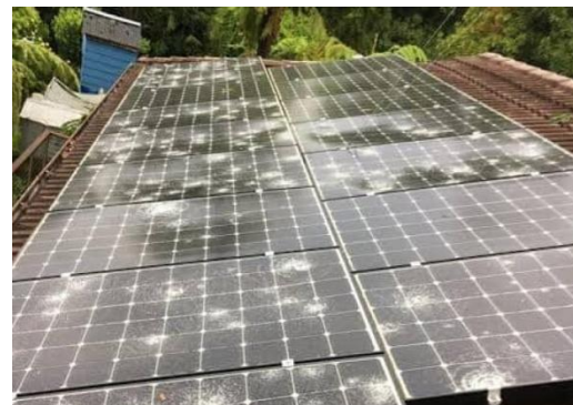
Solar panels damaged by hail
