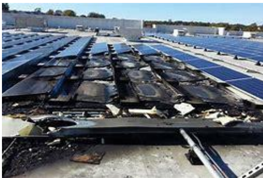
Remains of solar panels fire
