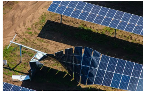
Oakey 2 wind damage
