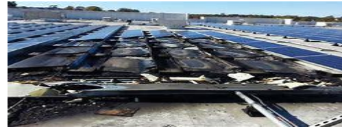
Fire damage to a PV solar IEGW
