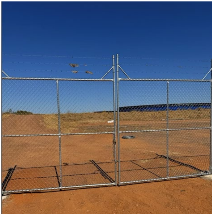
Exhibit 3 - 3.6-meter high-security fence with a barb wire top around the tanks located as a third inner fence which surround the tank containment area.
