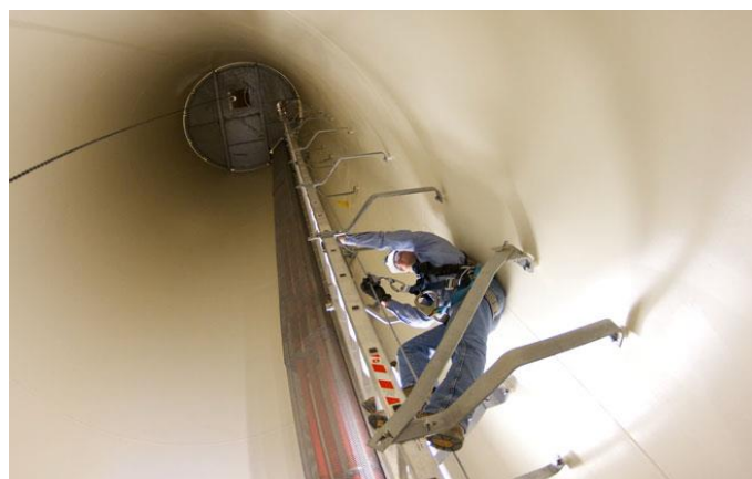
Figure 4- Ladder fixed to side of tower. Climbers back towards the side of tower
