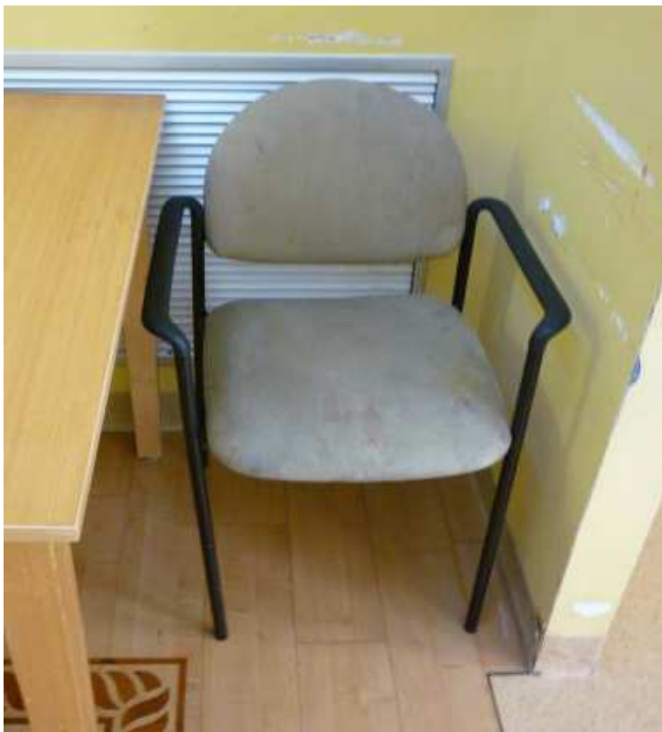
Image 8: Soiled Chair and damaged wall.
