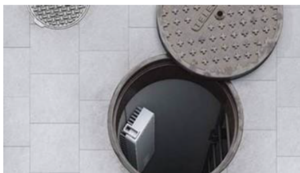
Figure 7: Future 5G small cell deployments, Top – antenna on street light pole; Bottom – base station equipment in access hole Courtesy, Ericsson
