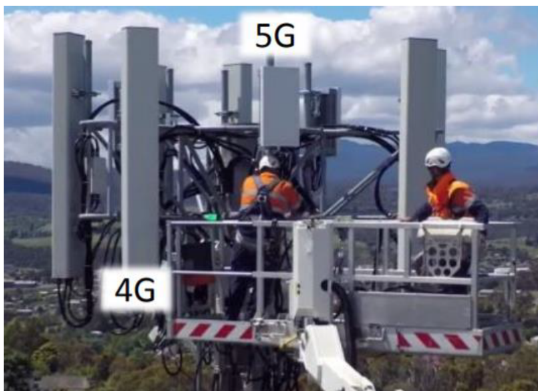
Figure 5: Typical 5G upgrade to existing base station.
