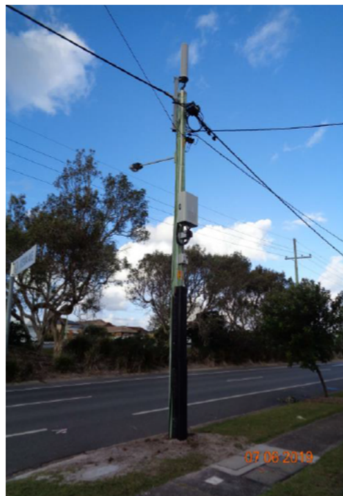
Figure 6: Current 4G small cell deployment on a street light pole
