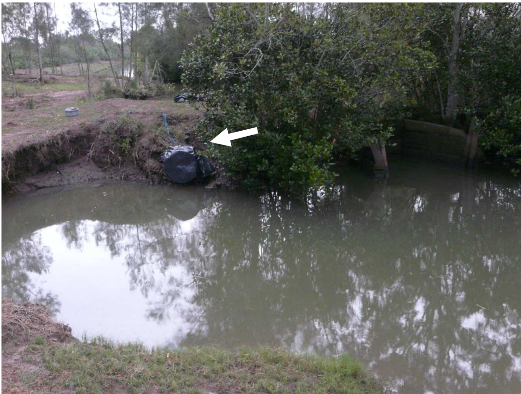
Figure 3. Reinforced plastic was placed over the overflow pipe (arrow) to prevent water escape.
