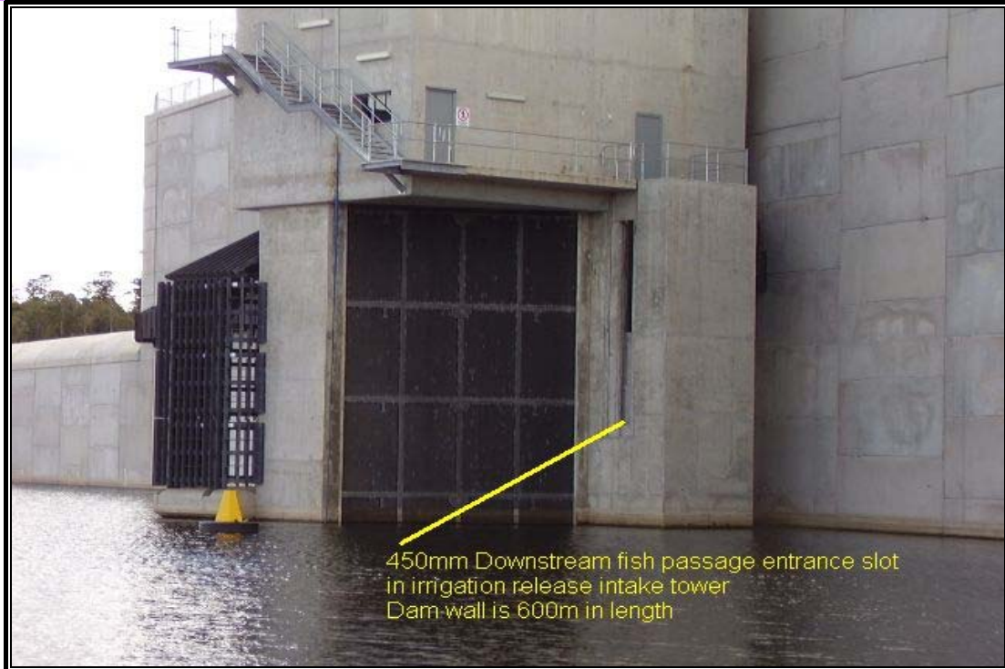
Image of downstream fish passage device attached to irrigation intake tower.
