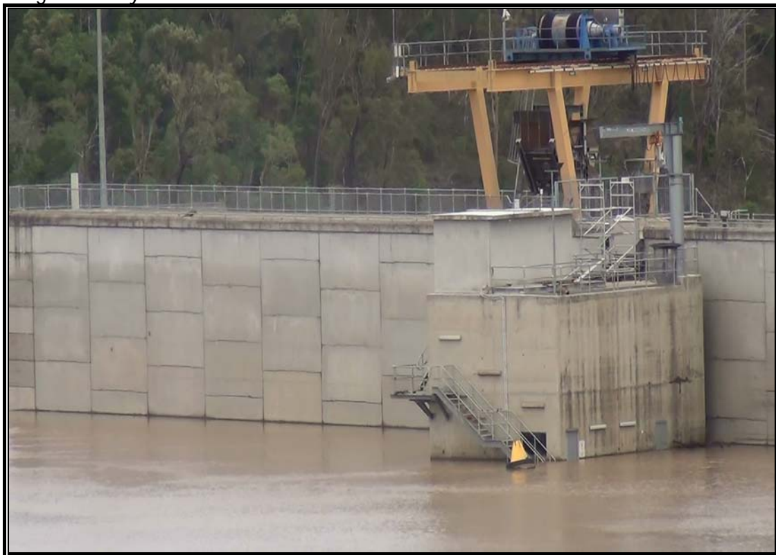
Image B taken 30 th Feb 2013 indicating flood level staining on control tower .
