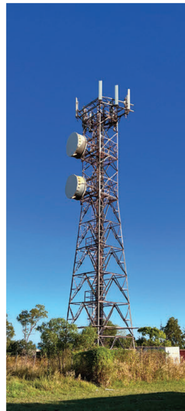
Mobile tower at Galiwin'ku
