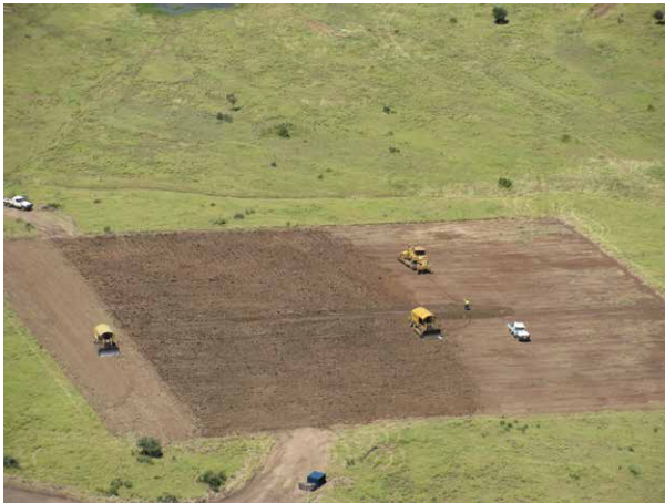
Construction of a lease area for a one-well pad (approximately one hectare).
