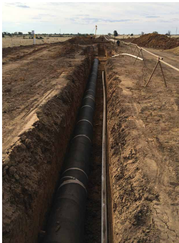
Fibre optic cable (right) lying alongside a gas transmission pipeline.
