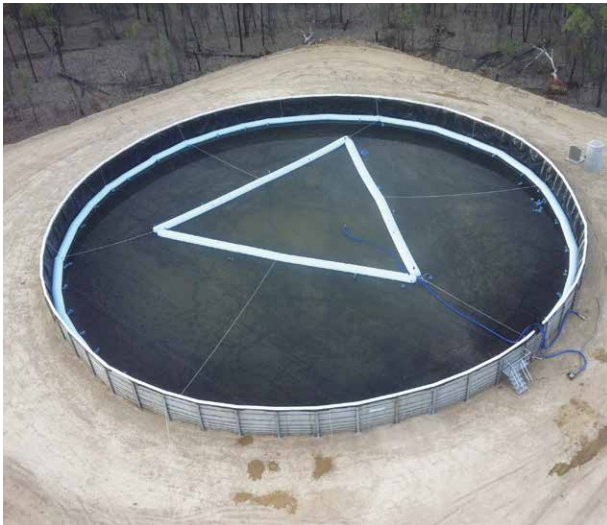
Completed 3.6 megalitre MOWST. The white triangle is a new water ballast system designed to maintain the integrity of the outer ring.
