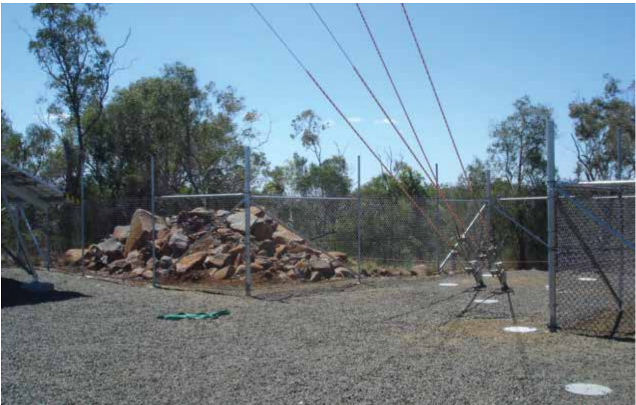
Guy wires used to stay a communications tower.
