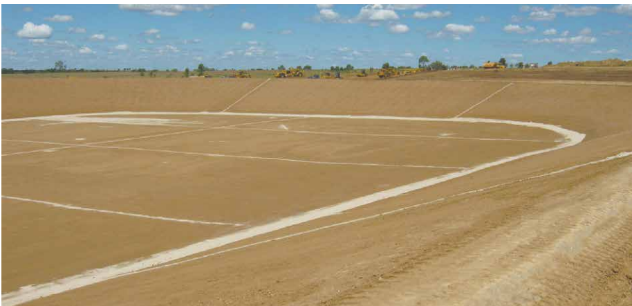
Drainage on the side walls of this WMP is designed to catch any leakage that may occur through the HDPE membrane.
