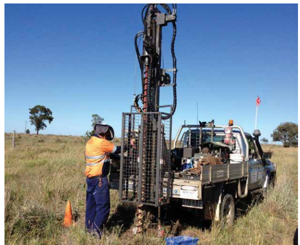
Typical truck-mounted drilling rig used to drill bore holes during geotechnical investigations.
