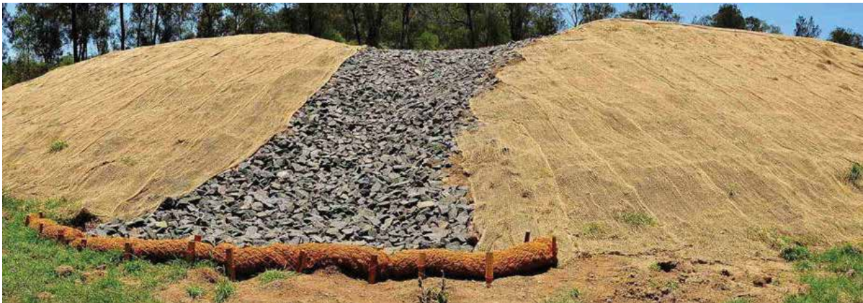
Rock lined chute batter that controls surface water and captures sediments coming off the pad during wet weather.
