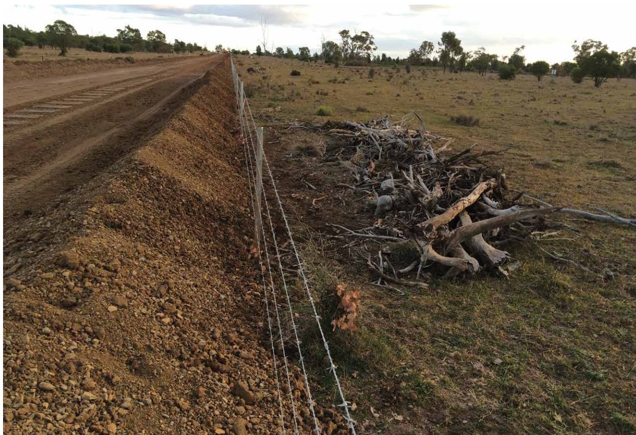
Clear and grade – topsoil on the left and sub-soil on the right with temporary fencing.
