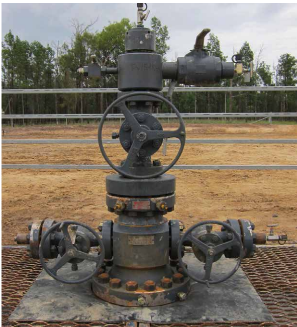
Completed wellhead with a Christmas tree (no pump required).
