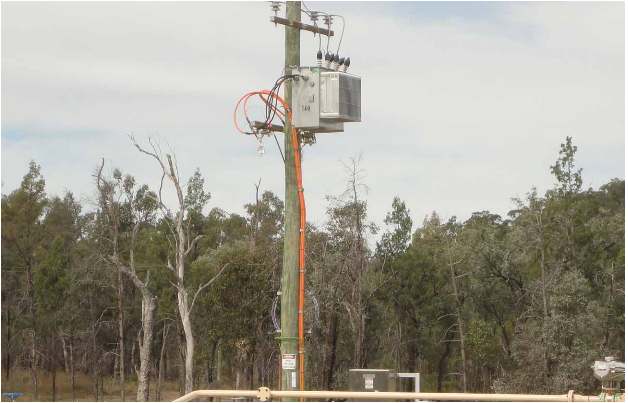
Example of a pole mounted transformer
