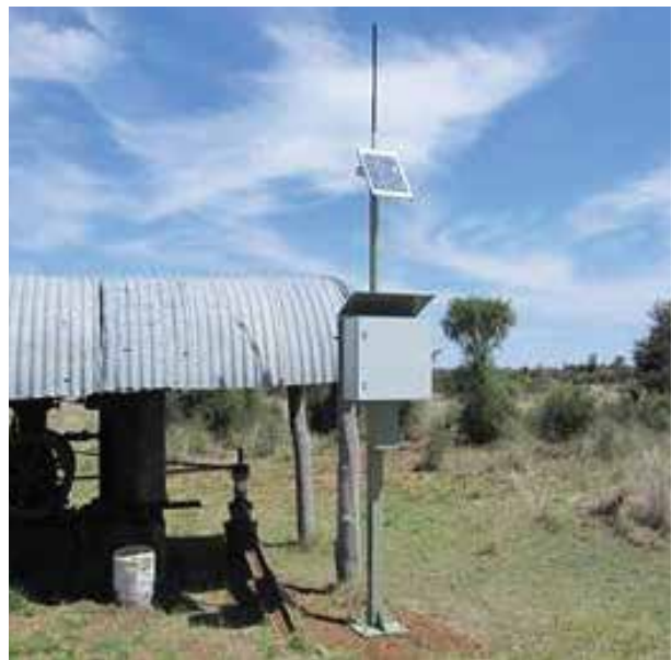
Telemetry station to the right of an existing landholder water bore.
