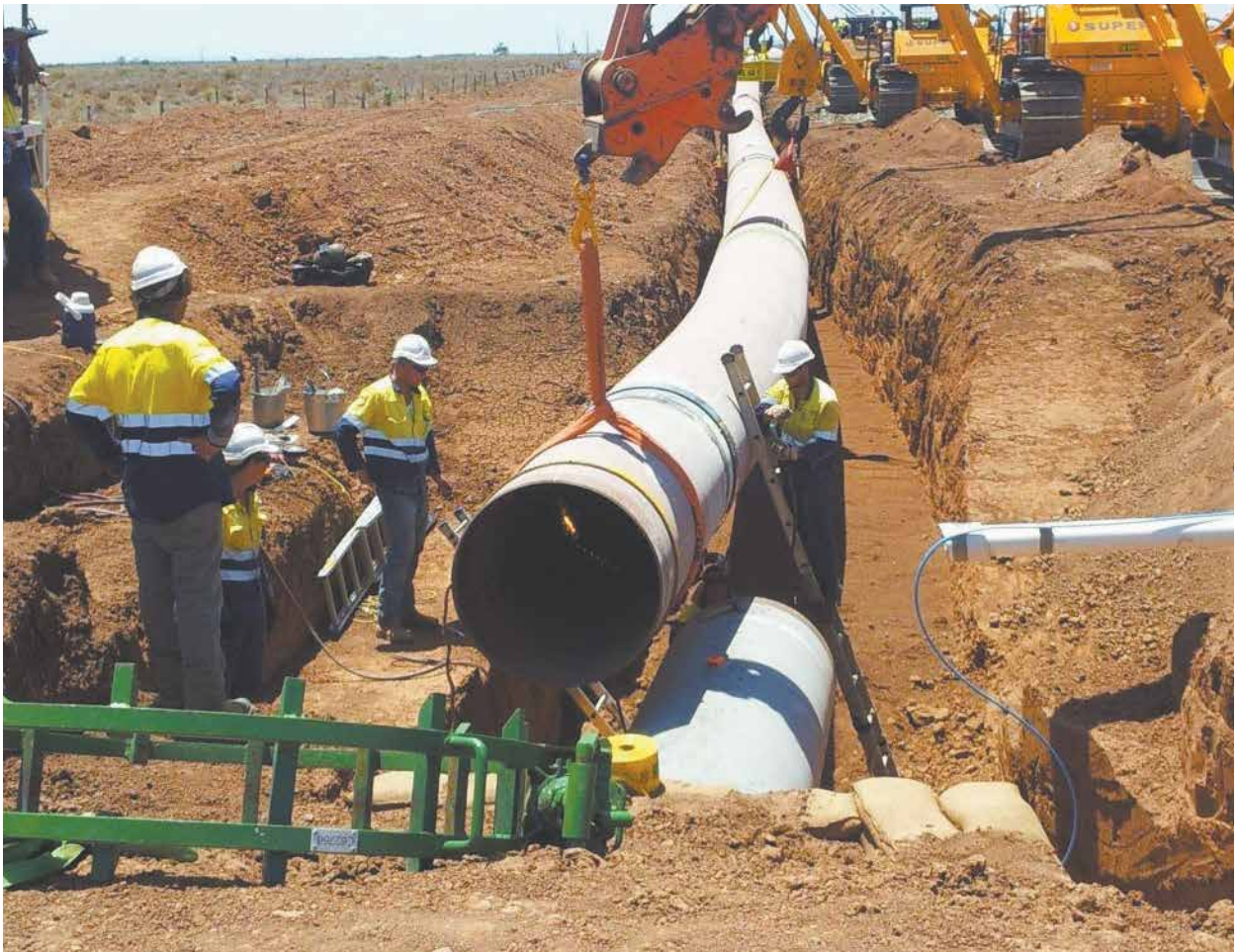
Tie-in welds are being used to join a section of welded pipe together.
