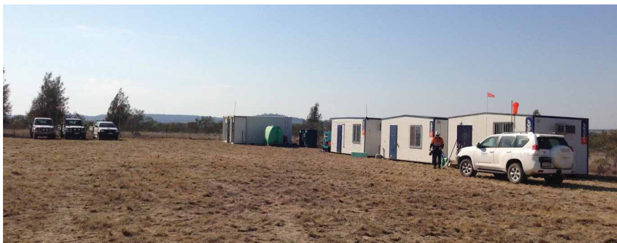
Typical site set-up – there are no flare pits and it occupies a much smaller disturbance area than gas production well lease.
