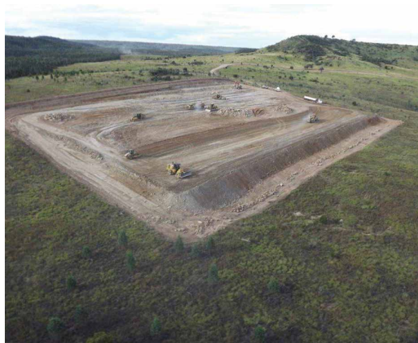
Construction of a lease area for a 10-well pad (approximately three hectares).
