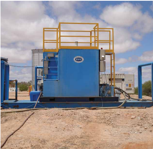
Sewage processing unit.
