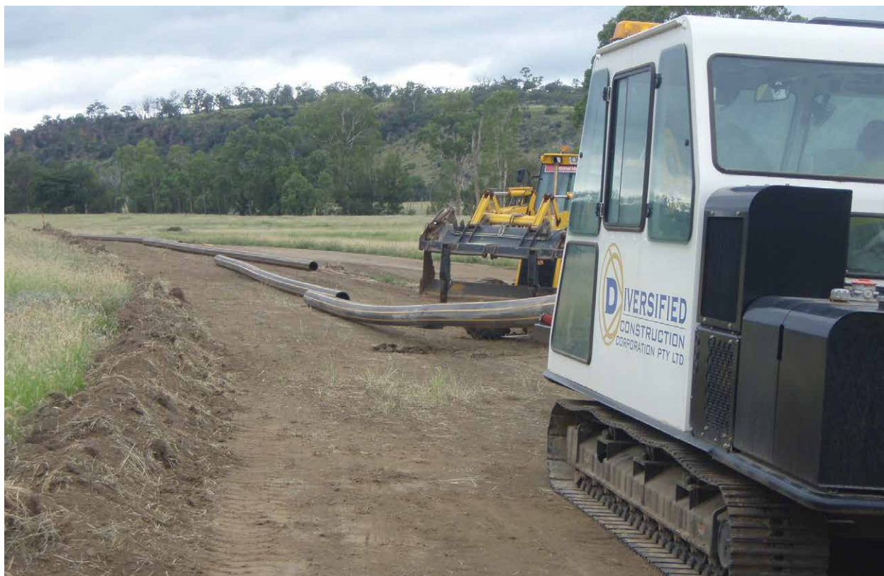
Water flowline stringing and welding. The machine in the foreground is a 'fast fusion' machine.
