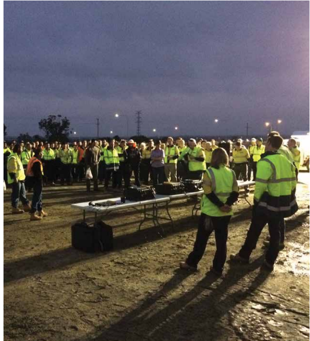
A tool box meeting held before construction commences on a gas transmission pipeline.
