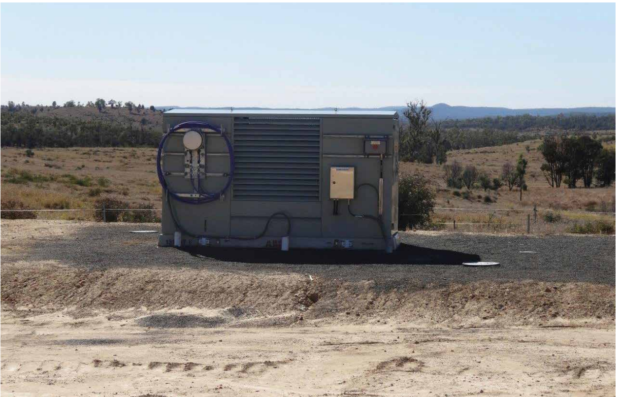
Example of pad mount transformer kiosk
