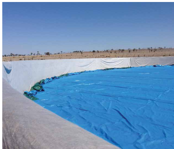
Liner installed in a MOWST.
