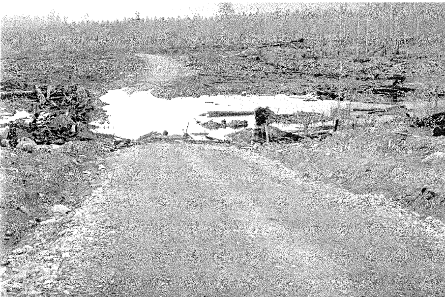
Figure 7. Road constructed through sinkhole, Florentine Valley, Tasmania, 2002, in breach of forest practices provisions:
