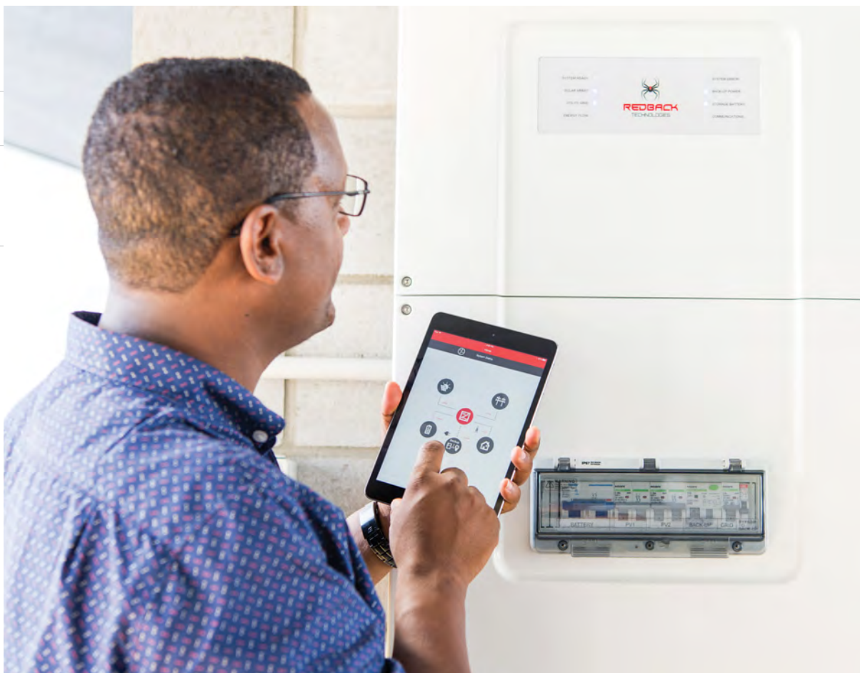
Australian firm Redback uses IoT and cloud technologies to help users manage solar energy generated onsite.
