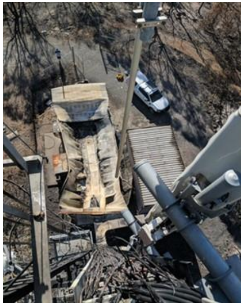
Figure 2: Fire-damaged mobile network facility, Mount Torrens SA
