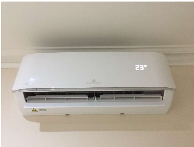
Figure 12 - Energy efficient split cycle air conditioning in every room
