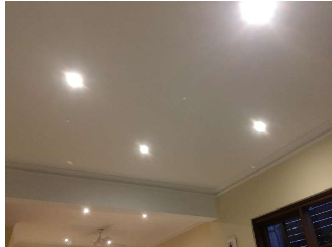
Figure 13 - Efficient LED lighting throughout
