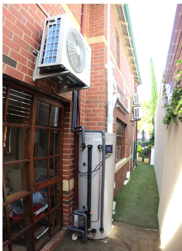
Figure 9 - Air Source Heat Pump for hot water
