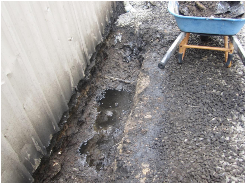
22.4 Figure 28: Completely non-compliant worksite oils, fuels and other vehicle fluids leaking into unsealed pit
