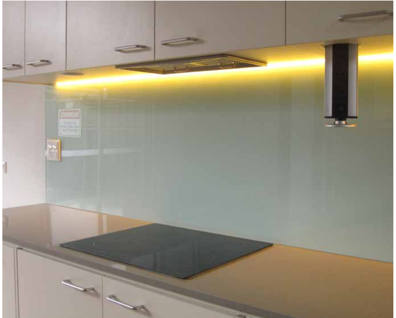
Pull-down GPO unit, Mission Australia (Victoria) housing, MSM Architects.
