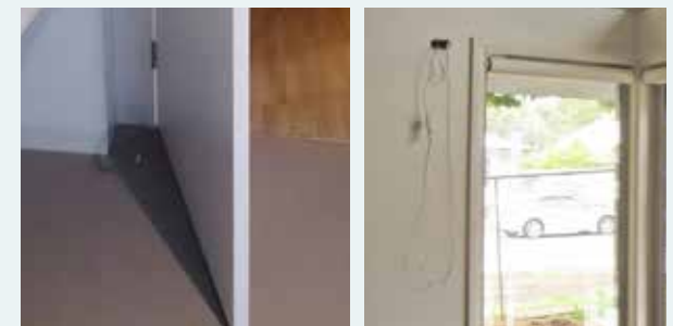
Slimline wall corner guards and timber-look vinyl flooring, Abbotsford (left) and pre-wiring for future blind automation prior to install of coverplates, TAC RIPL Housing (right).
