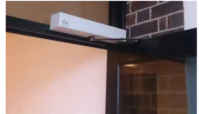
Automated apartment doors, showing internal wall button for automatic door opening (above), and typical door automation hardware (below), Abbotsford.
