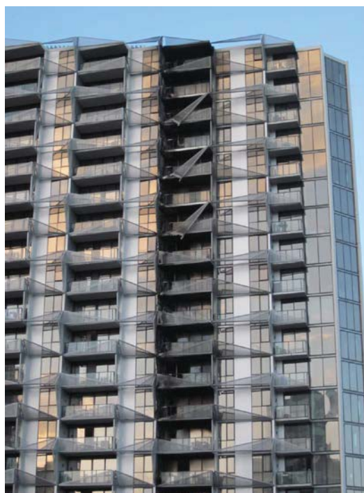
Photo Post Fire
