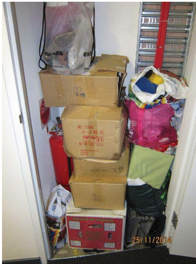
Figure 13 - Fire extinguisher cupboard on Level 6.
