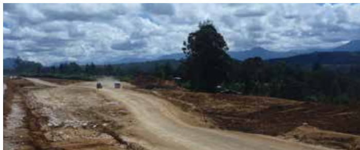
Runway extension work next to Tari Airport, 2011. Photo credit: James McIlraith/University of Otago.
