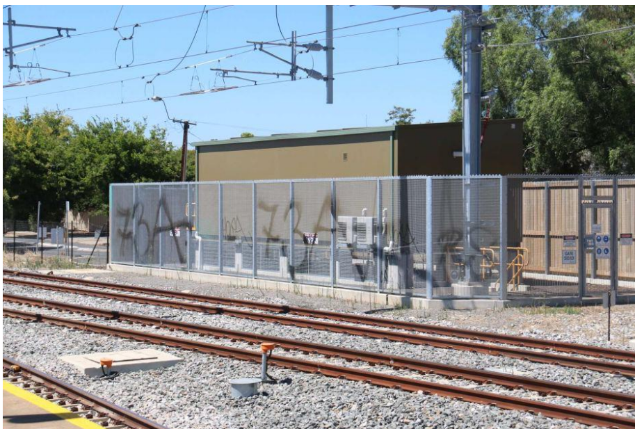
Electrical substation next to SA's Seaford railway line where Robin Johnson Engineering used asbestos containing material for the flooring. (ABC News)
