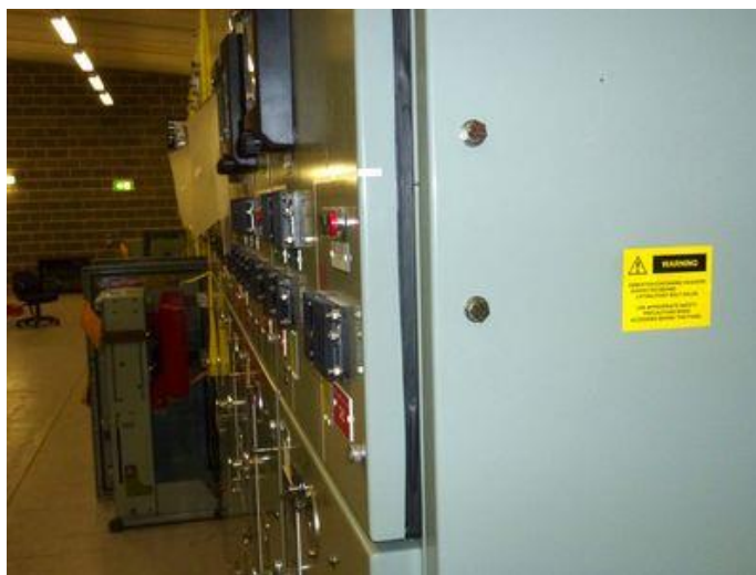
Electrical switchgear equipment inside an Ausgrid substation
