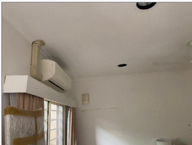
Timber pelmets have deteriorated due to the location and leakage.
