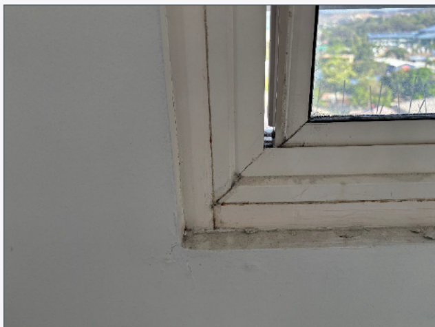
Window seals are failing across the majority of units.
