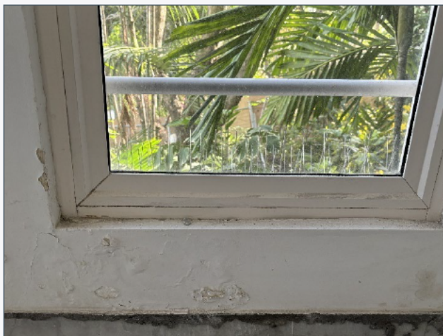
Damage resulting from non-watertight windows.
