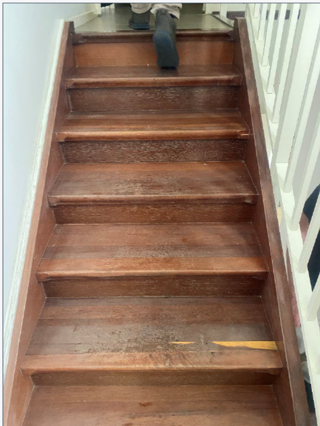
Stairs have worn finish and damage.
