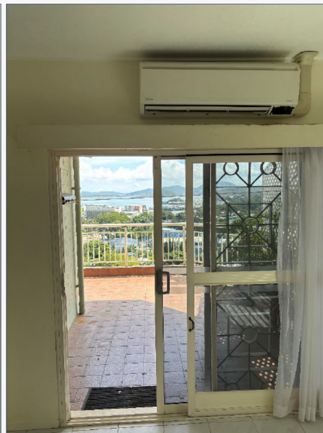
View of existing indoor AC unit from kitchen with damaged pelmets
