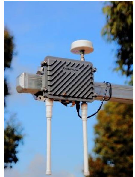
Figure A2: Roadside infrastructure for vehicle-to-infrastructure communications
