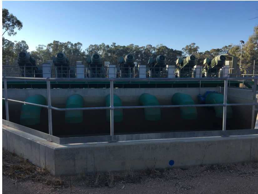
Pumps at Chalka Creek in the Hattah Lakes area
