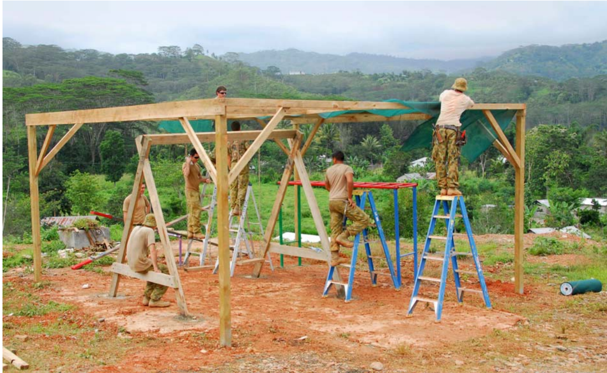
Engineers from the 3 Combat Engineer Regiment, as part of Timor-Leste Battle Group 3, build a playground for the children of the Hope Orphanage in Gleno (image courtesy Department of Defence).
