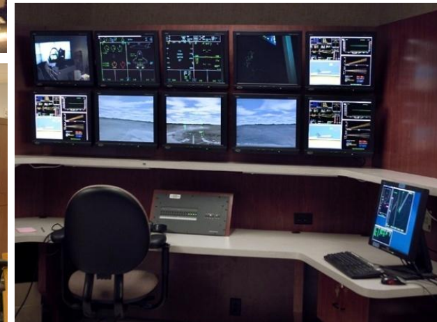
VIF Fixed Base Control Room
