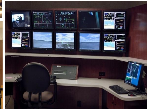
VIF Fixed Base Control Room
