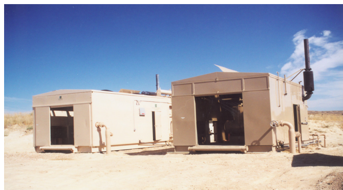
Photograph of typical CBM field compressor station
