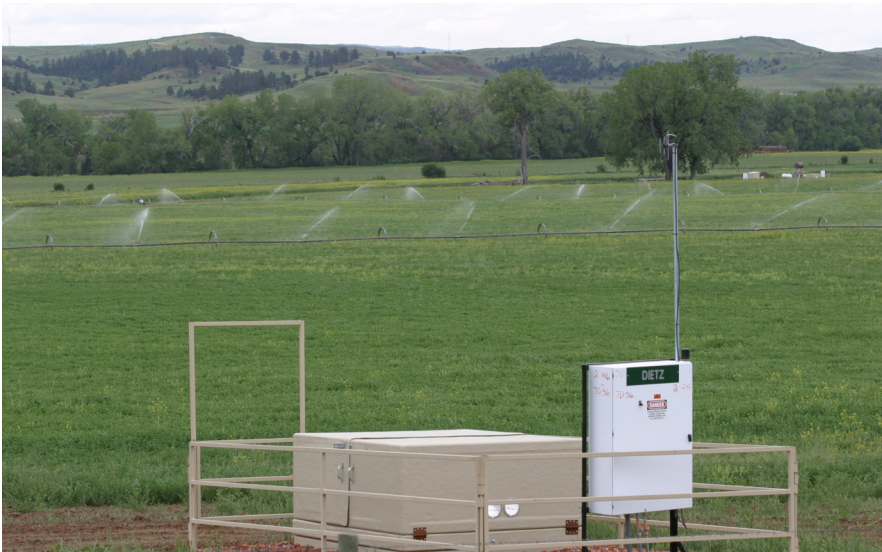
CBM well head equipped with radio monitoring system and field irrigation in background, Wyoming
