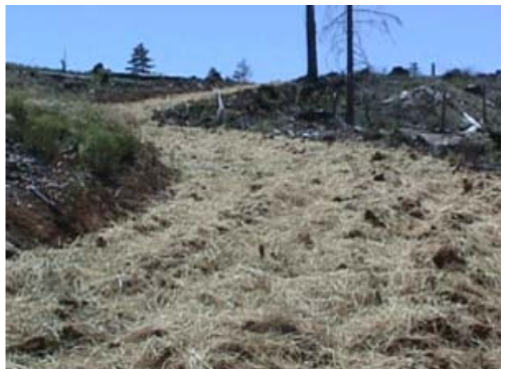
A road decommissioned by ripping, mulching, and seeding. Mulching as Best Management Practice to reduce soil erosion and control the infestation of noxious weeds. Photograph provided by BLM, Coos Bay District
