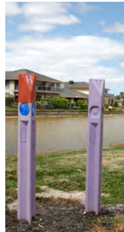
Above The Sandhurst Club, located just outside of Frankston in Melbourne's south east, uses purple pipes and recycled water to reduce its dependence on mains water supply
